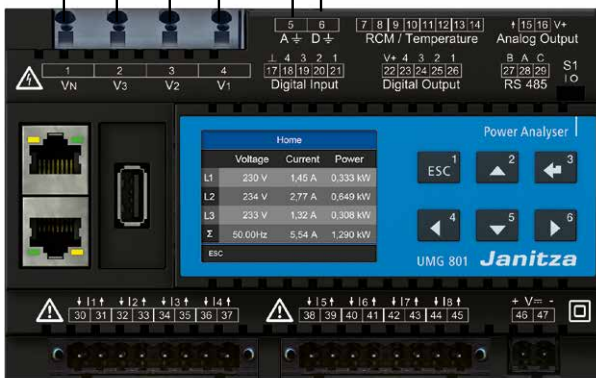
Fig. Connection example for "voltage measurement". PELV
